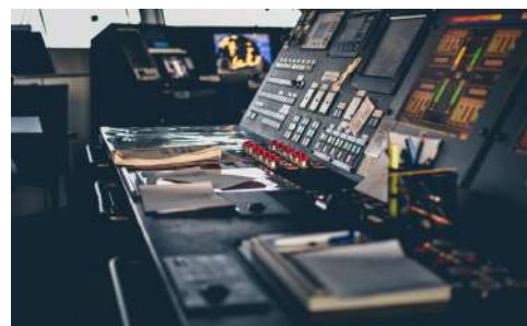
Railway Signaling & Train Control Systems
