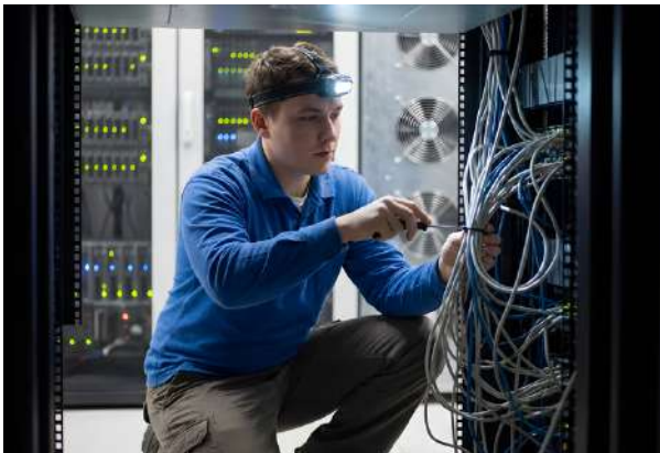
Server Rooms & Data Centers
